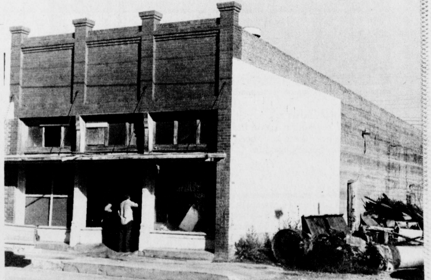
FACE-LIFTING —This building, which has housed many businesses down through the years, is being renovated for the teen center. Among possibly others, businesses in this
