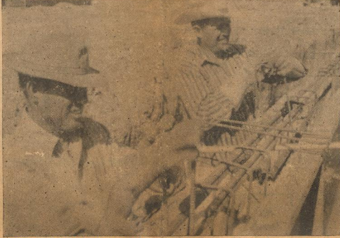
UNDER CONSTRUCTION in west Dimmitt is the new eighty-thousand-square-foot high school building. Workers building supporting structures for the foundation are Jim Hudson (left) and Van Alsop (right) both of West Texas Builders, Lubbock. See story. —Cowan photo
