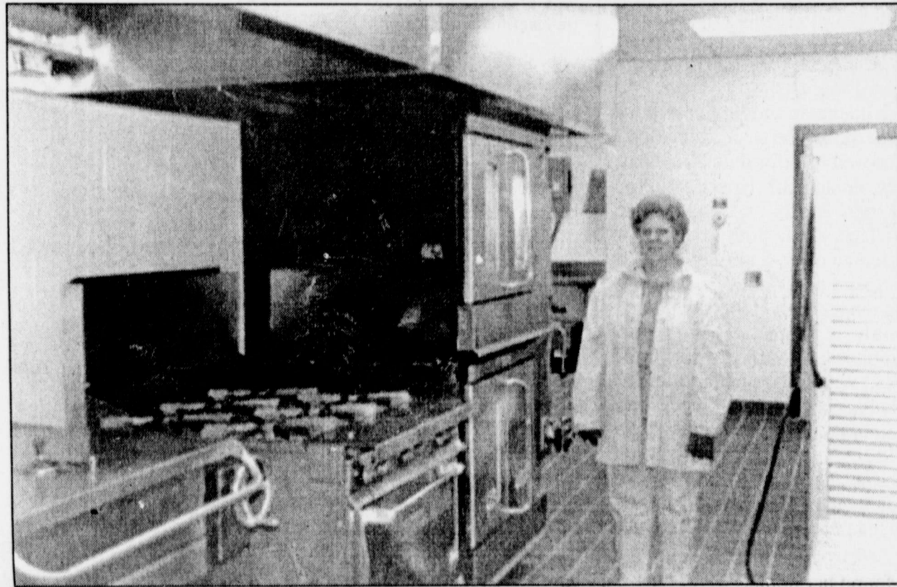
NELL BALLARD, WISD cafeteria supervisor, stands by her new state-of-the-art cooking equipment. Nell and her talented cooking crew were finally able to move into the new cafeteria on Wednesday and served the first meals on Thursday.
