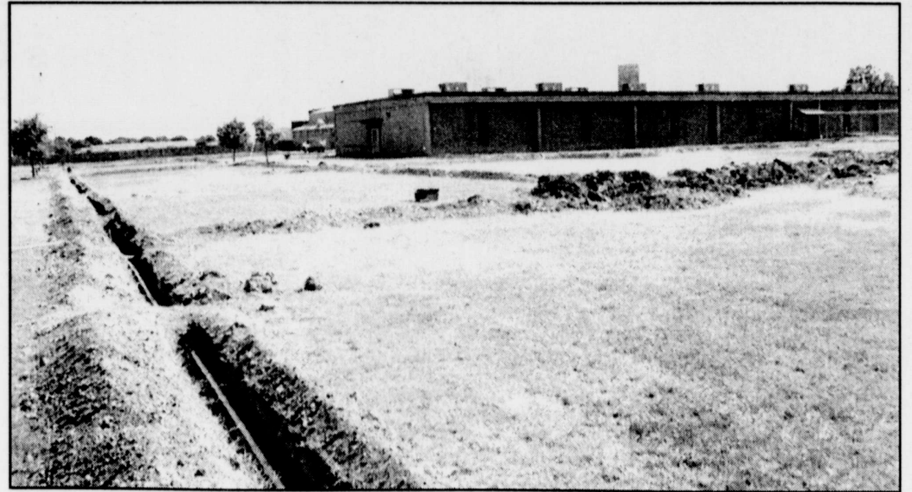
SPRINKLER SYSTEMS are currently being installed on the elementary grounds as another step to improve school properties. Sprinkler systems have already been installed in many areas and, according to school maintenance supervisor Dale Montgomery, plans are to install the efficient watering systems throughout the school grounds with work being done by school personnel.
