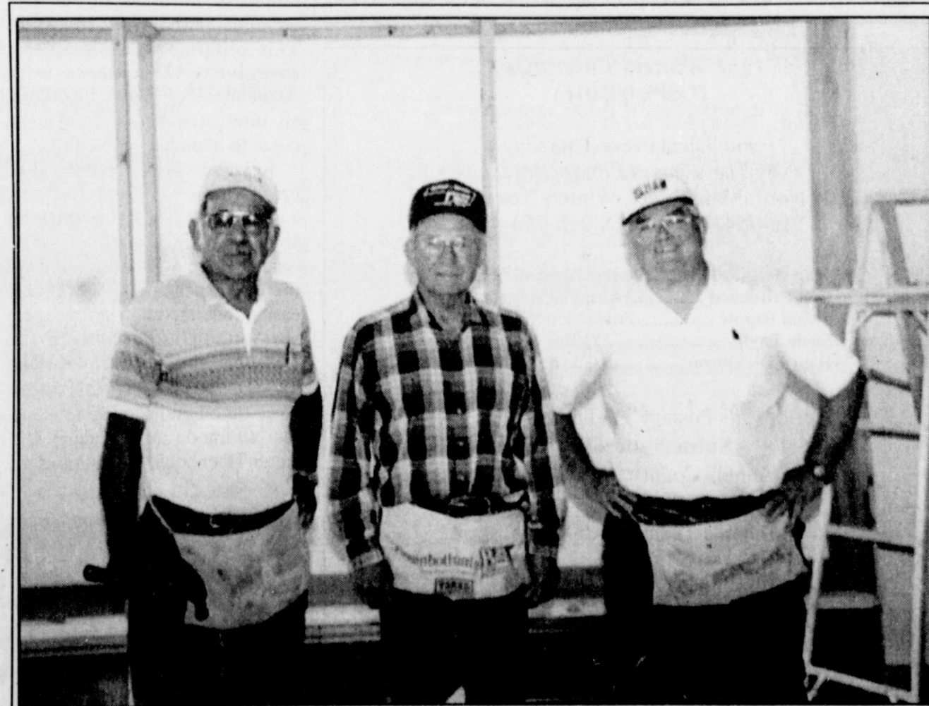
THESE TALENTED VETERANS, Louis Delacruz, Robert Holder and Billy Ray, have been busy building seven display cases in the Veterans' Room of the Rock Hotel. The 4'x8' cases with glass shelves and storage drawers will house military memorabilia.
