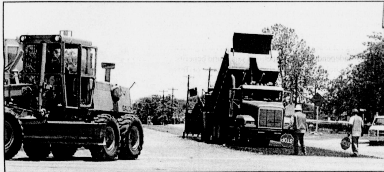
NEW ROAD SURFACE has been installed for fifteen miles beginning at the intersection of Hwy. 83 and FM 1770 which passes by the football stadium, track field, and city park, in addition to housing additions. Construction is being done by Brannon Paving of Victoria, Texas.
