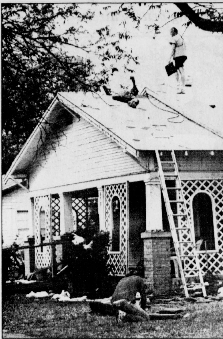
QUITE A FAMILIAR SIGHT around Winters are scores of roofers trying to repair and replace most of the roofs in town which were destroyed in the hailstorm of May 24.
