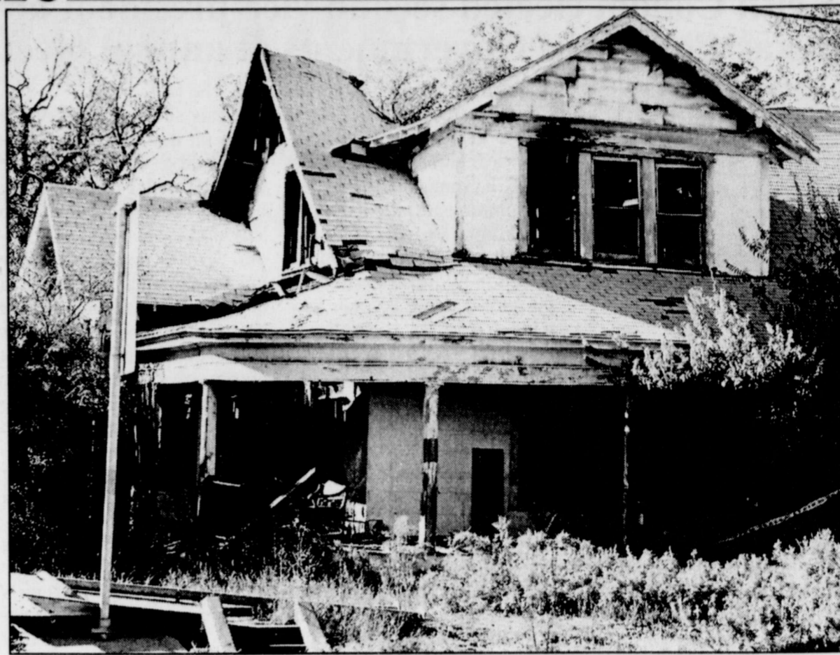
STILL WAITING to be demolished are the charred remains of this two-story house in the 300 block of North Main. The home of Lynn and Oscar Medina was destroyed by fire on February 26, 2002, and soon after condemned. City Manager Aref Hassan says he has been unable to make progress on demolishing the structure due to lack of commitment and agreements from BFI Waste Systems and the Texas Commission on Environmental Quality (formerly TNRCC), which dictates proper disposal of materials. Hassan says, however, that he is still pursuing all these avenues to clean the dangerous eyesore.
