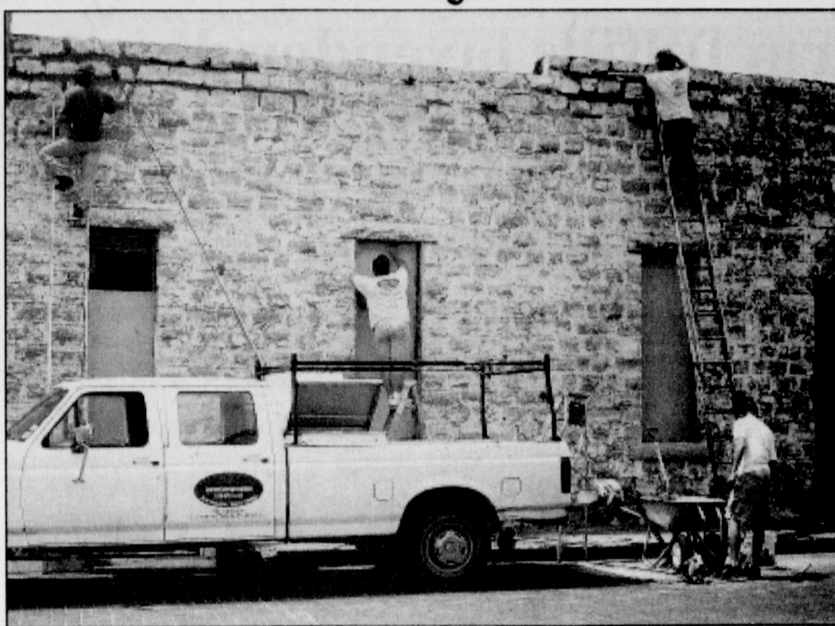
GETTING A NICE FACELIFT is the wall on the West Dale side of Raymond's Clip Joint. The back portion, which has been painted, belongs to Dean Burns. Workers replaced mortar and painted the wall with a rubber type paint. The remaining portion of the wall belongs to Raymond Lindsey who says he has no immediate plans to paint his portion.
