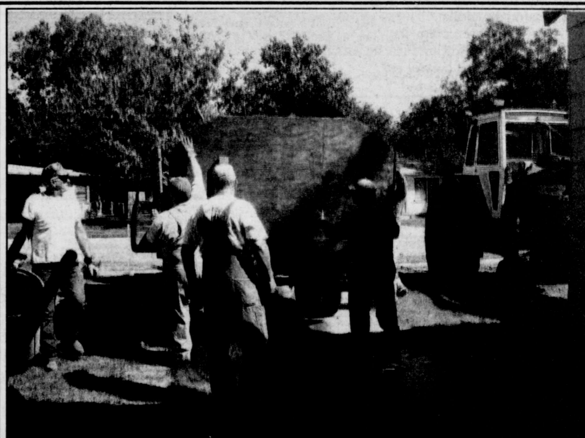
BUSY FRIENDS worked last week to clean and repair the home of Don Dunstan who broke his neck while working on his roof about five weeks ago. Recent heavy rains further damaged the roof and destroyed sheetrock and insulation inside the home. Workers include (l-r) Charles Brewer, Mike Neal, Hank Bourdo, and Jim Lincycumb who provided the truck, Alan Cooper provided and operated the front-end loader at right. (photo by Jean Boles)
