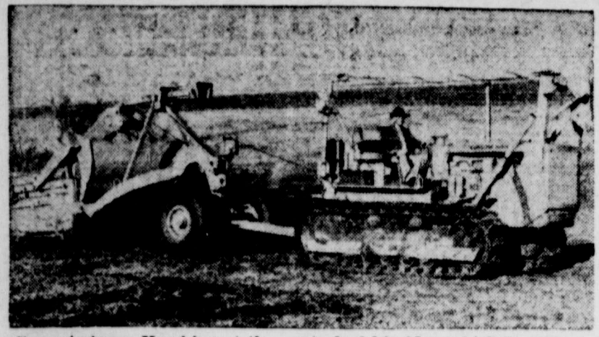
Commissioner Hawkins at the control of his idea which is storming Oklahoma as improving county roads without cost to taxpayers or county.
