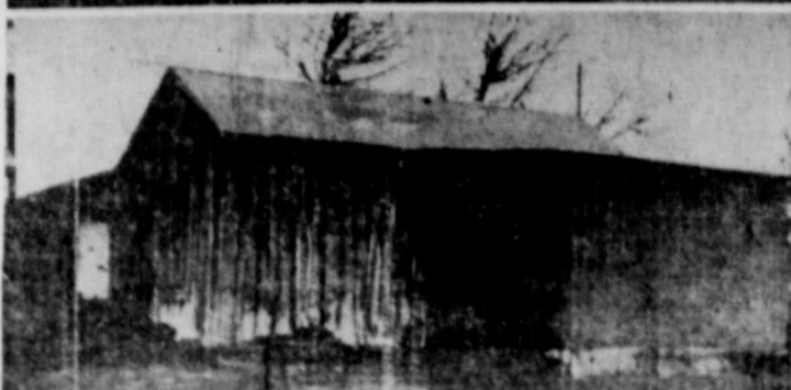
To create the new house, top, from an original homestead, the owners added new rooms, reroofed with colorful asphalt shingle and put on asbestos siding. Several new windows were added.
