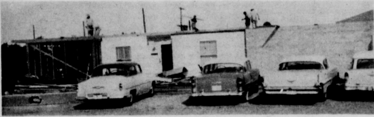
KINDA DAMP OUT (AND IN) —Workmen took the roof off the John Harris Clinic early this week, as part of the remodeling and rebuilding program now underway at the local institution. The clinic is being doubled in size, with new space for the laboratory, another doctor's office, consultation room, and other offices. The front and north side of the structure will be finished in brick, while the south side will be attached to the hospital.
