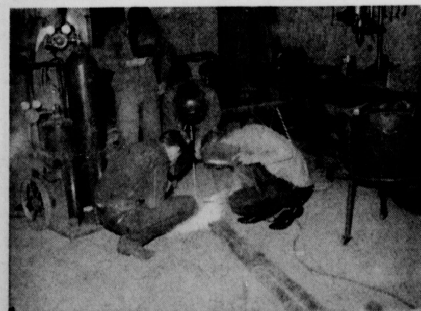
JERRY SCOUTCHEN, right, has plenty of help using the electric welder to cut a length of pipe.
