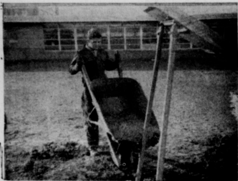
RUDY PHILLIPS dumps a load of cement to hold a slide firmly in the ground.
