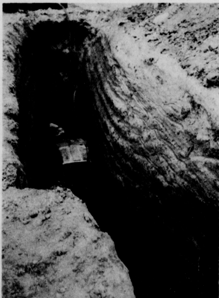
A GOOD VIEW — The above photo shows the machine at work which was used to bore a hole under U. S. Highway 277 to accommodate part of Bronte's
