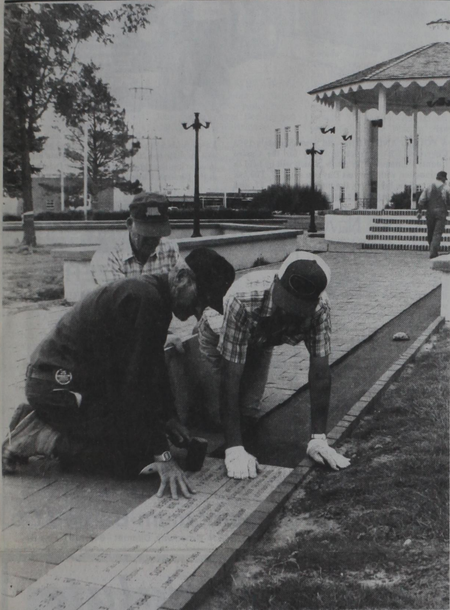
TILE LAYING UNDERWAY —Centennial Plaza Project Chairman Robert Hawkins (foreground) gets a helping hand from Bill Birdwell and Dale Winders (right) in fitting red-granite commemorative tiles along a walkway Saturday morning. In background is Willis A. Hawkins. Volunteers sorted and fitted almost 300 tiles Saturday and are working this week to prepare the "tile beds" for
