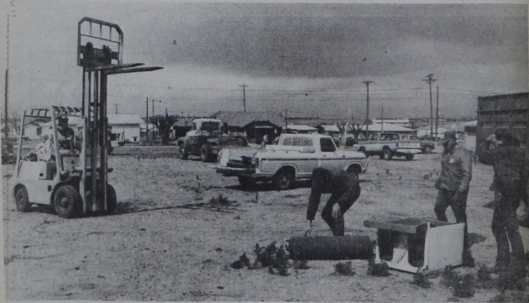
GRUNT-LIFTING AND FORK-LIFTING —Volunteer workers combine brawn and heavy equipment to clear away old appliances, foundation slabs, tree trunks, debris and weeds
