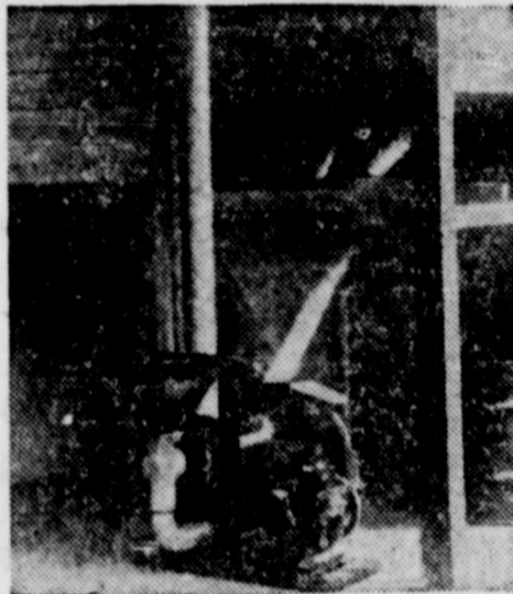
This blower-equipped hammer mill can be fed from overhead bins and later re-elevate the ground feed into adjoining bins, located over the mixer.
