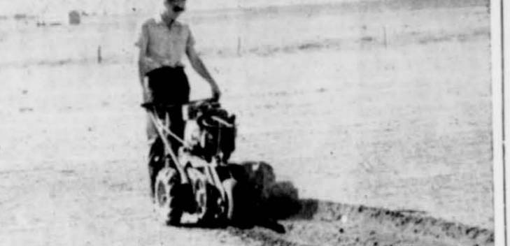
MAKING USE of the portable ditch digging tractor is Burrus McRee. He is making the cross ditches for the installation of gas lights on the Dimmitt airstrip. See story.
