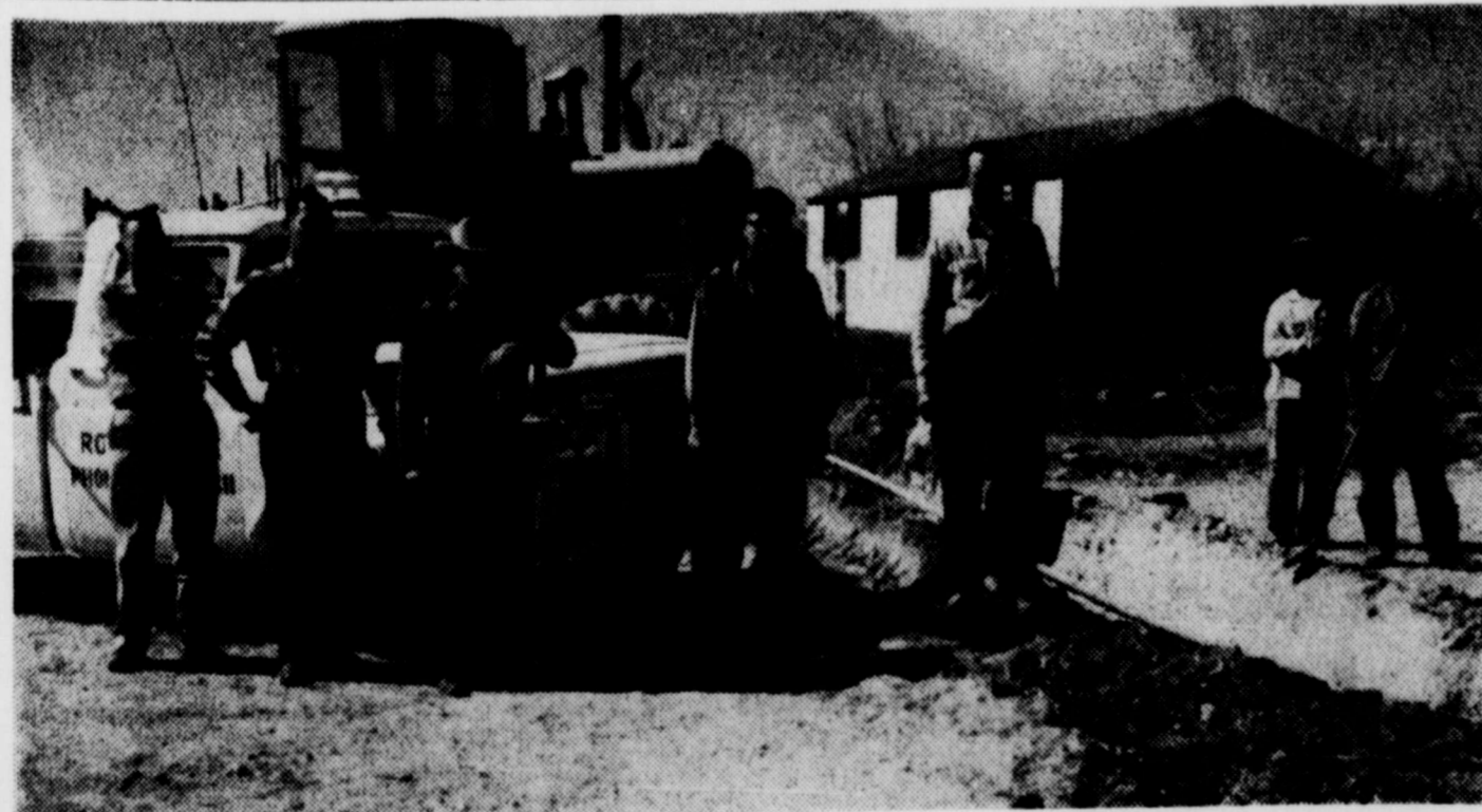
REPLACING CITY WATER LINES—Thousands of feet of new water lines have been laid throughout the city of Robert Lee. Most of the work has been done ahead of the paving. Many old lines were rusted out and were too close to the surface of the earth. A Precinct 1 maintainer was used to scoop out trenches for the pipe. Shown in the above photo are (left to right) Cecil Mayfield, water supt., Mayor W. D. McAdams, Commissioner Fern Havins, Jett Hood, maintainer operator, Ed Trimble, who has been working with Mayfield for some time, and Santos Tiperina and Jessie Torres, members of the ditching crew.
