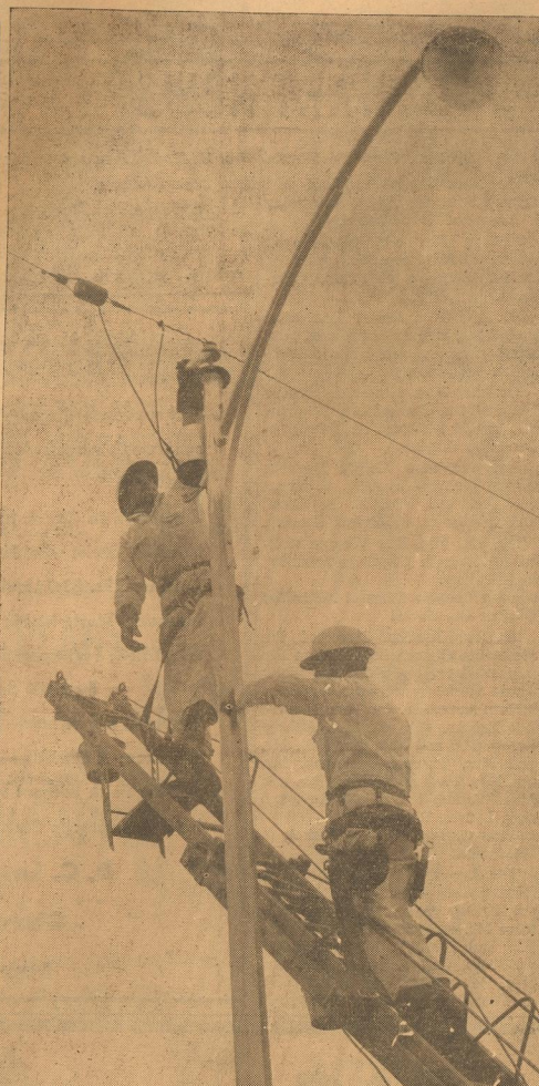
POLE PAINTING —Southwestern Public Service employees began this week their regular paint-up of city street lights. Arthur Wockack (top) probably had the coldest job in town when this photo was taken on the Square Wednesday. Below him is another Southwestern Public Service employee from Plainview, Charlie Hayes. They were assisted by Floyd Keeling and Bob Burns in their uncomfortable, but appearance-improving work. — News photo
