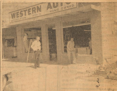
FACELIFTING IS STARTED —as Vade Kirby (right background) and an employee of Plainview Plate Glass and Mirror (left background) tear out old bricks in order to put in a new complete-glass front. Larry Allen (foreground), manager of Western Auto Store is shown looking the situation over. —Mickey staff photo
