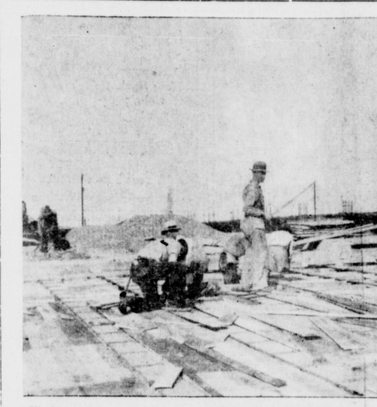
Workmen here are shown building forms for the flooring of the new overpass at Eighth street and Katy railroad, which is nearing completion by the Jensen Construction company. The structure, one of the most beautiful in the state, will be opened about June 1. It carries the new route of Highway 80, the Bankhead, over the Katy tracks where once a small wooden bridge spanned the tracks.
