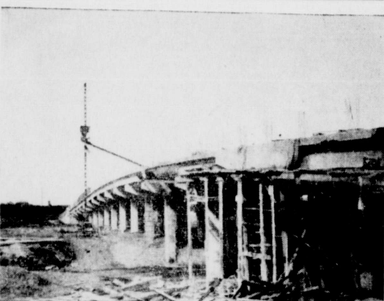
Here is a view of the new overpass carrying Highway 89 over the Katy railroad tracks on East Eighth street. Something of the magnitude of the $125,000 structure is shown.
