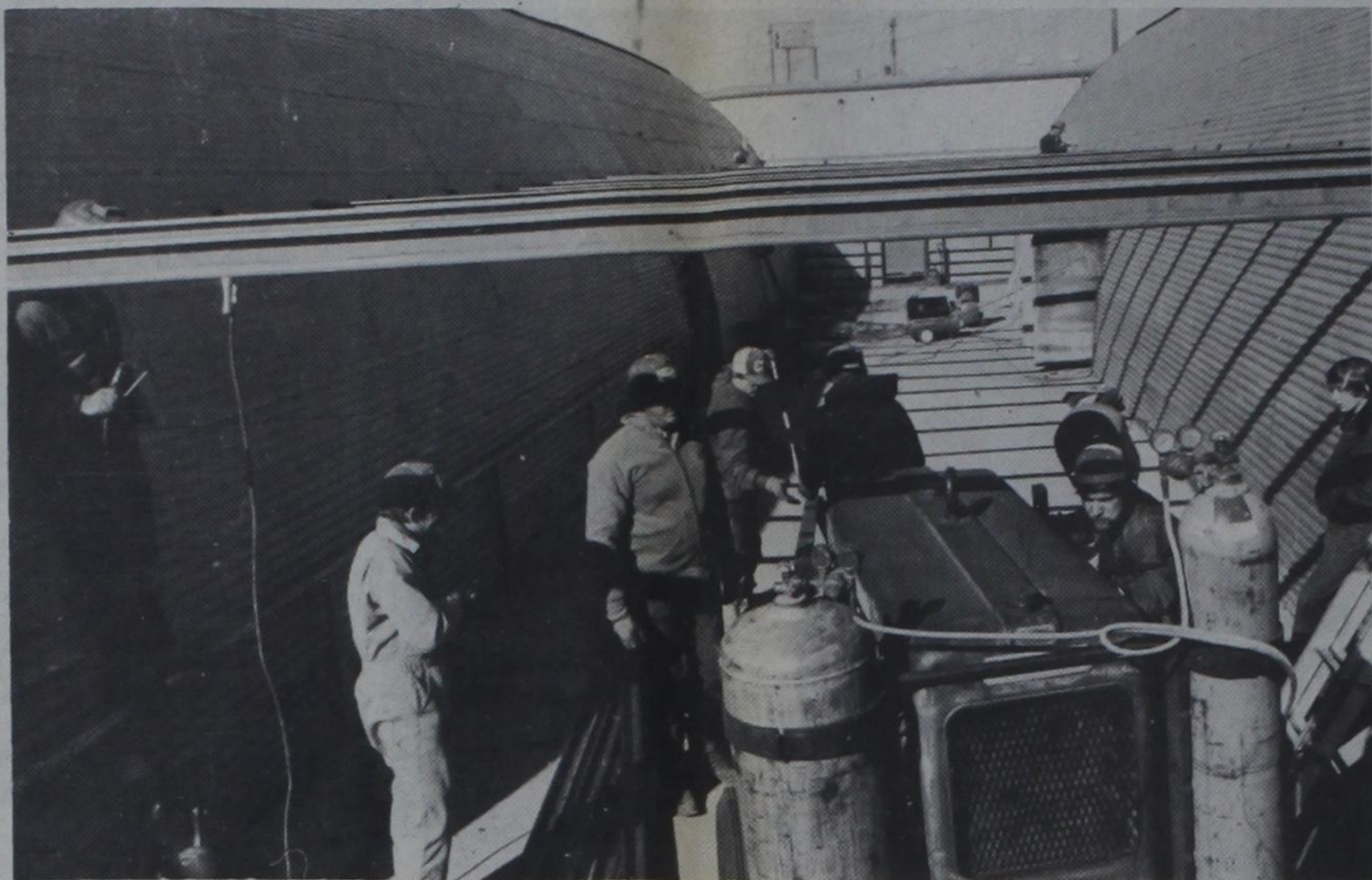
A COVERED WASH RACK and more hog pens will be available to the county's youngsters at the Junior Fat Stock Show this year, thanks to this project by the Dimmitt Young Farmers, who conduct the annual show. Here, the Young Farmers put up the steel roof beams Saturday for a weather
