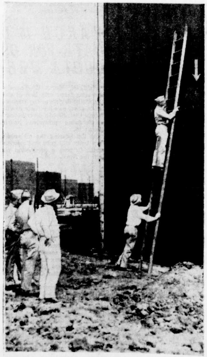
DAMAGE INSPECTION AT ARUBA—U. S. Army officials inspect shrapnel dent (arrow) in oil tank at Aruba Island off Venezuelan coast following sub attack on tankers and shore points.
