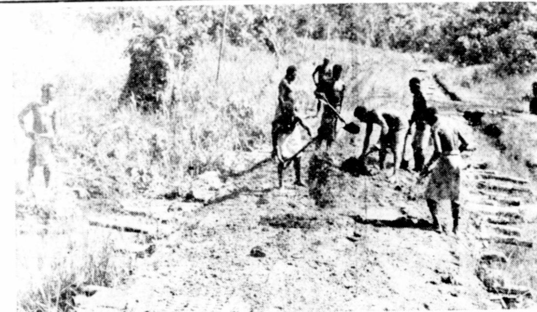
MODERN JUNGLE TRAIL —New Guinea natives repair an American corduroy road that leads to an advanced base, somewhere on the island. Road, flanked by underbrush, is ready to carry anything from a jeep to a convoy of transport trucks.
