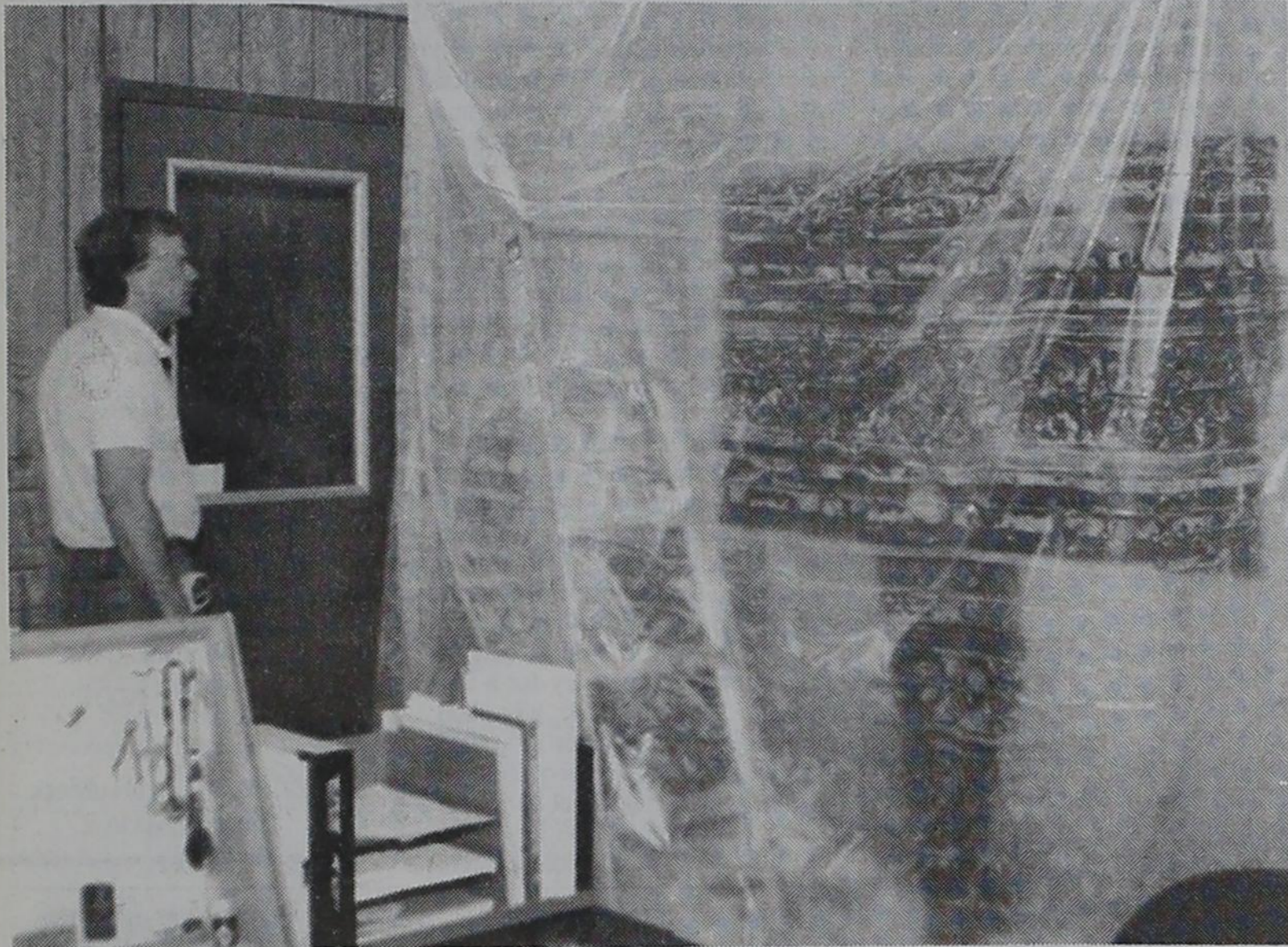
IT'S NOT A GHOST — That's Keith Hoelting under the plastic sheeting, as remodeling work begins in the Castro County Sheriff's Office in the courthouse. Hoelting and his assistant, Darren Keys, are installing a window for the new consolidated dispatcher's room, which will house the
