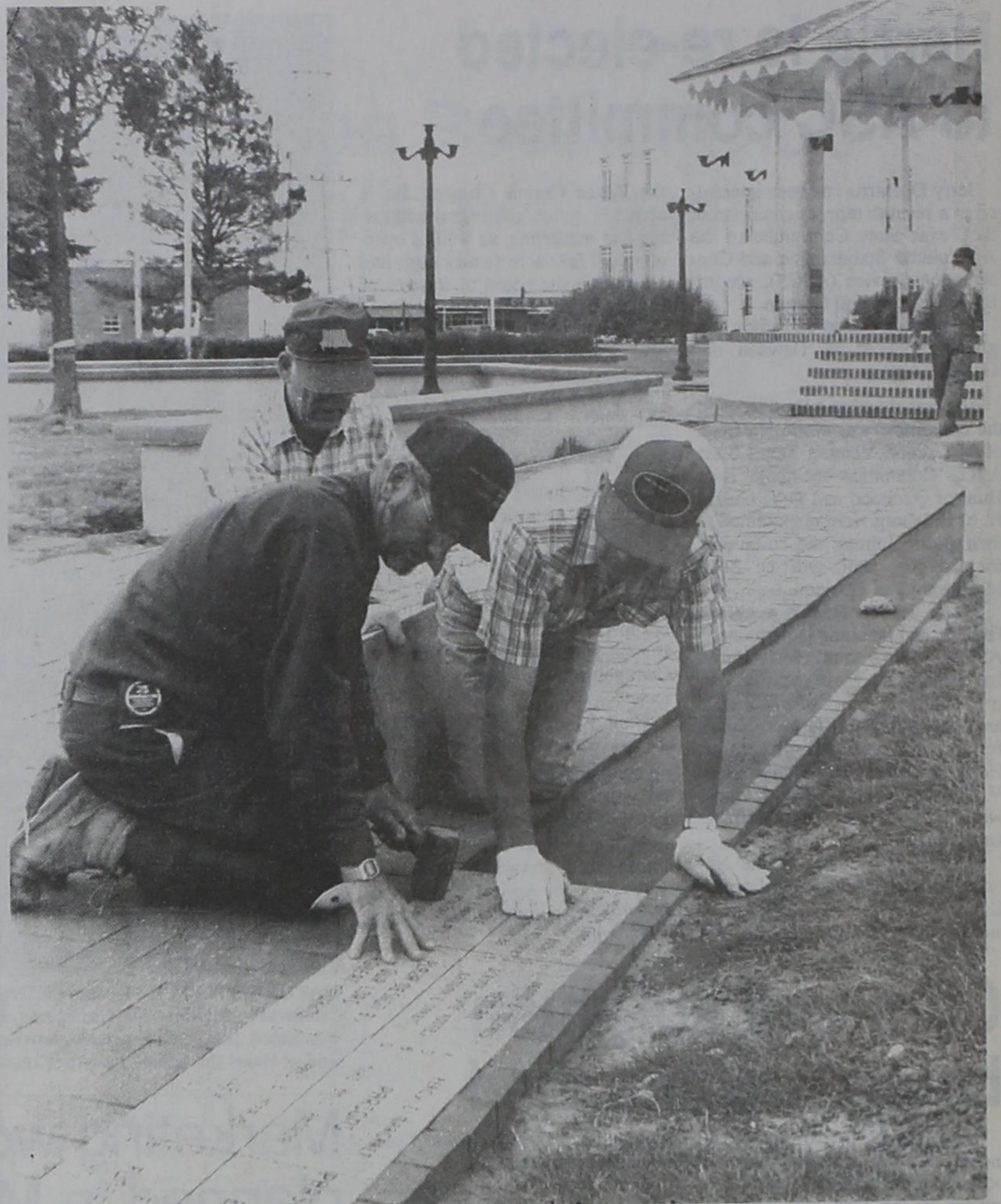
TILE LAYING PARTY — Centennial Plaza Project Chairman Robert Hawkins (foreground) gets a helping hand from Bill Birdwell and Dale Winders (right) in fitting red-granite commemorative tiles along a walkway. In background is
