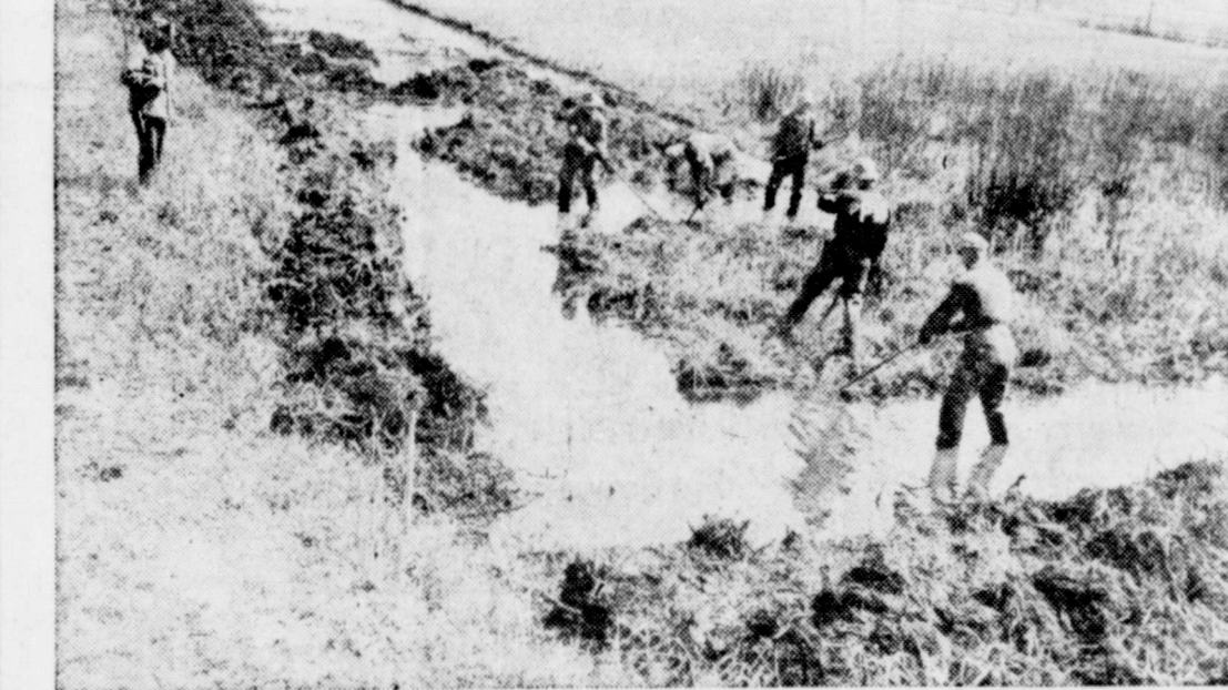
POW'S HELP CRANBERRY GROWERS—German prisoners of war, assigned to help cranberry growers in Wisconsin, arrange marshy ground to form dikes around new beds. When pond freezes it is covered with sand. In spring thaw, sand settles to form bed where cranberry vines are planted. POW's receive 80 cents in canteen coupons and 50 cents from U. S. Treasury per day.
