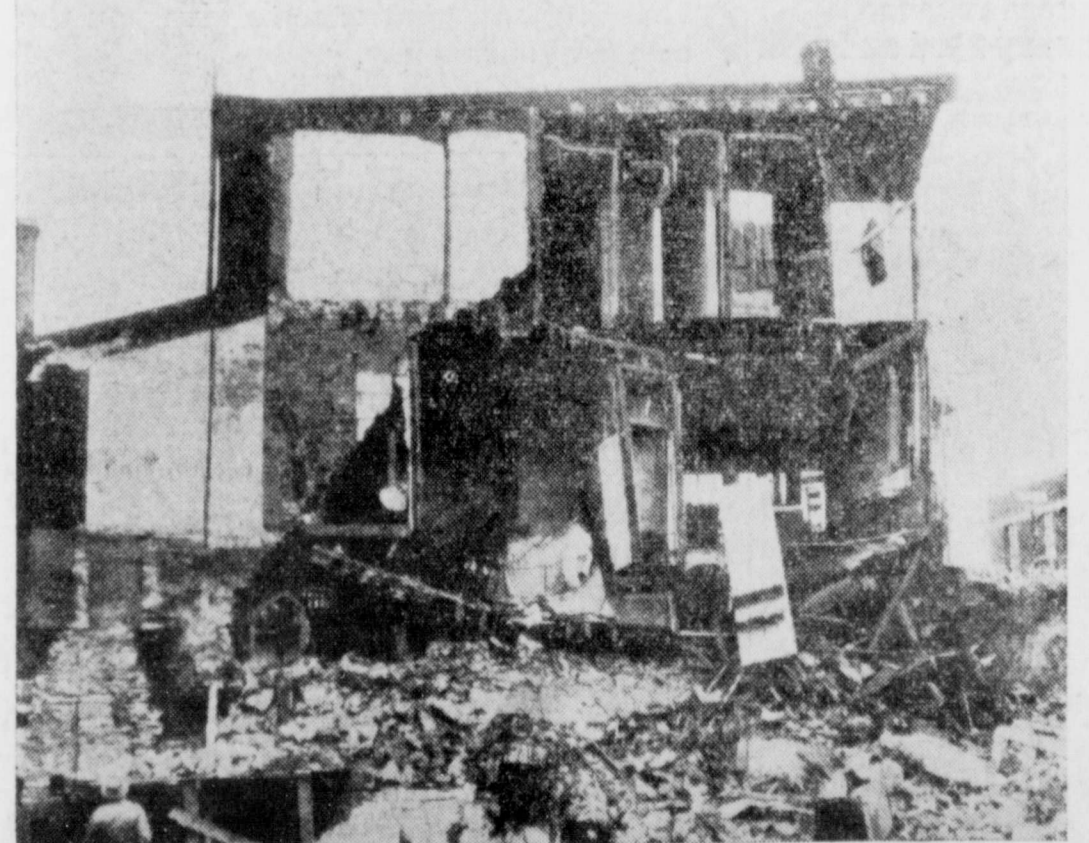
TOO CLOSE —The rear wall of this building collapsed into an excavation that had been dug too close to its foundation in Tacony, Pa. Although a restaurant was on the lower floor, no one was injured.
