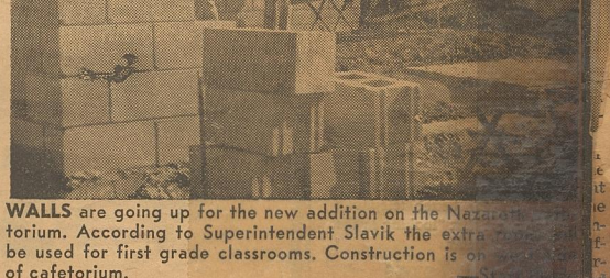
WALLS are going up for the new addition on the Nazareth school building. According to Superintendent Slavik the extra space will be used for first grade classrooms. Construction is on of cafeteria. —Staff Photo
