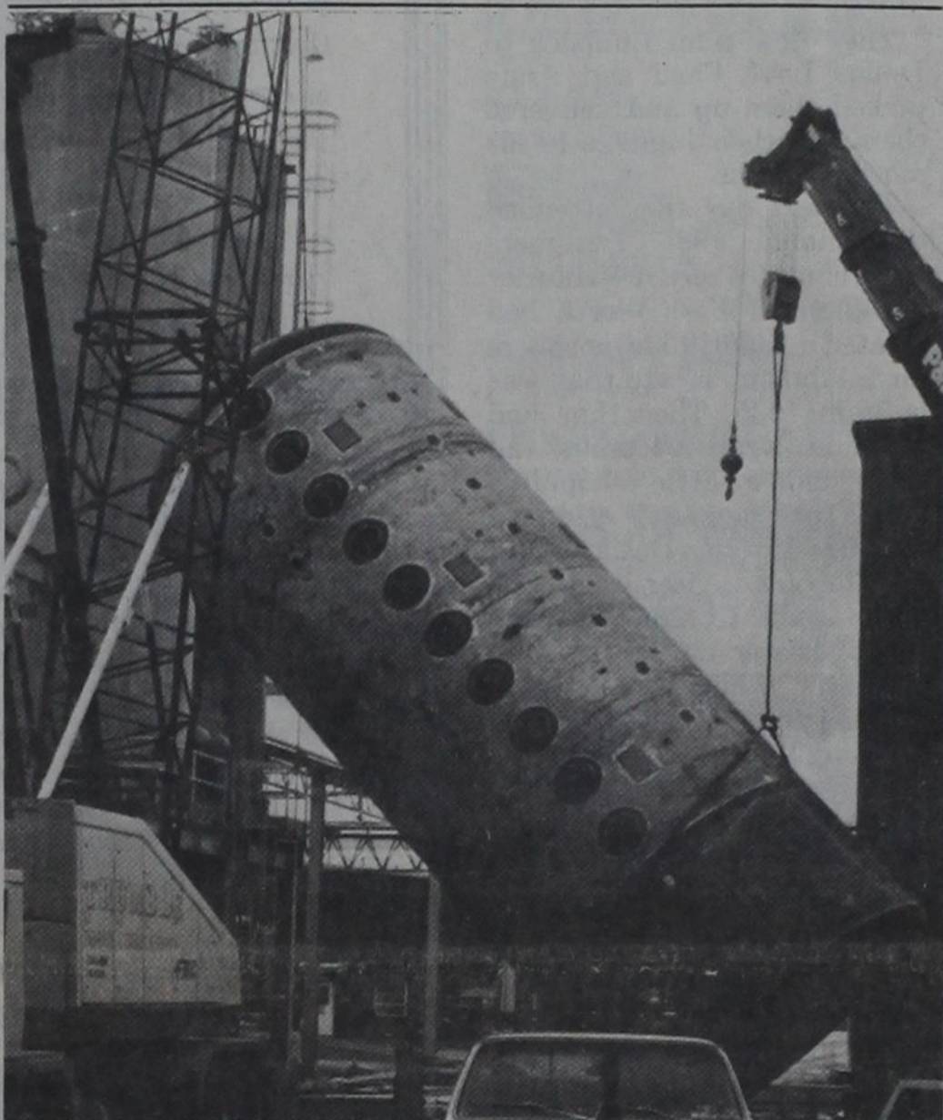
THE LEANING TOWER OF FRUCTOSE —Workmen from Trumble Construction Co. of Lubbock raise a 55-ton tank Friday during construction work at American Fructose Corp. The tank was transported from Minnesota on a special 11-axle trailer rig on a 7-day journey. The tank has 2½-inch thick walls, and is just one of several large tanks that will be installed in the expansion project, which will continue through early 1986.
