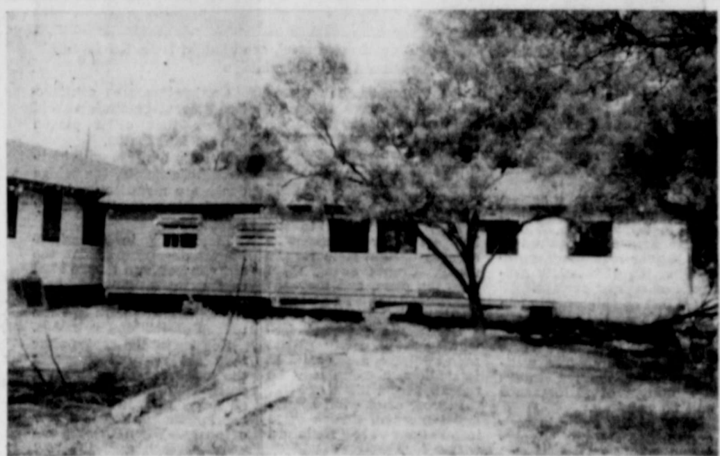
NEW ANNEX IN PLACE: Shown above is the new annex which has been moved into place at Teen Town, butting up against the back of the main building to form a "T". The annex was once used as a field house at Bulldog Stadium. Work is to begin soon on connecting it to the main building and putting the finishing touches to it. It will increase the size of Teen Town's recreation area almost half, and also provide a kitchen for the Mothers Club which is sponsoring the new addition. Several hundred dollars are yet to be raised to pay for the work. Many free hours of free labor and material have already gone into the project. Capps Photo.
