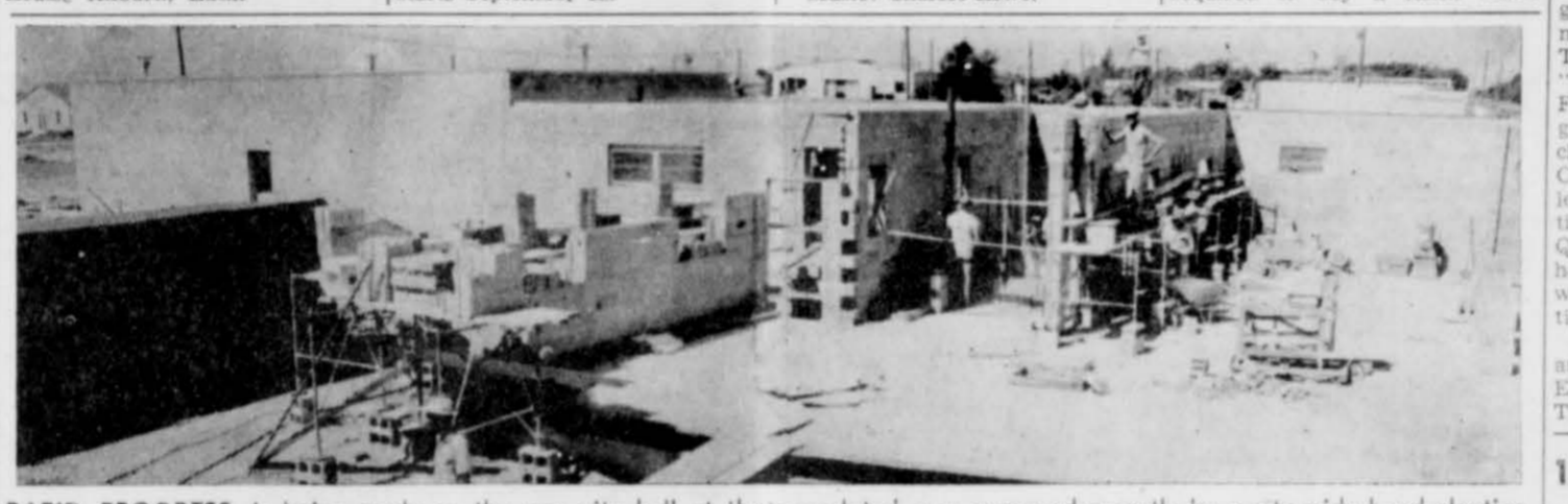
RAPID PROGRESS is being made on the new city hall at the corner of southeast second and Jones Street. The walls are rapidly taking place and an early fall completion date is planned. The new city hall, expected to cost more than $90,000 when completed, was approved recently by a city-wide bond election. It will be one of the finest in the area, replacing the outgrown city hall located on east Bedford.
