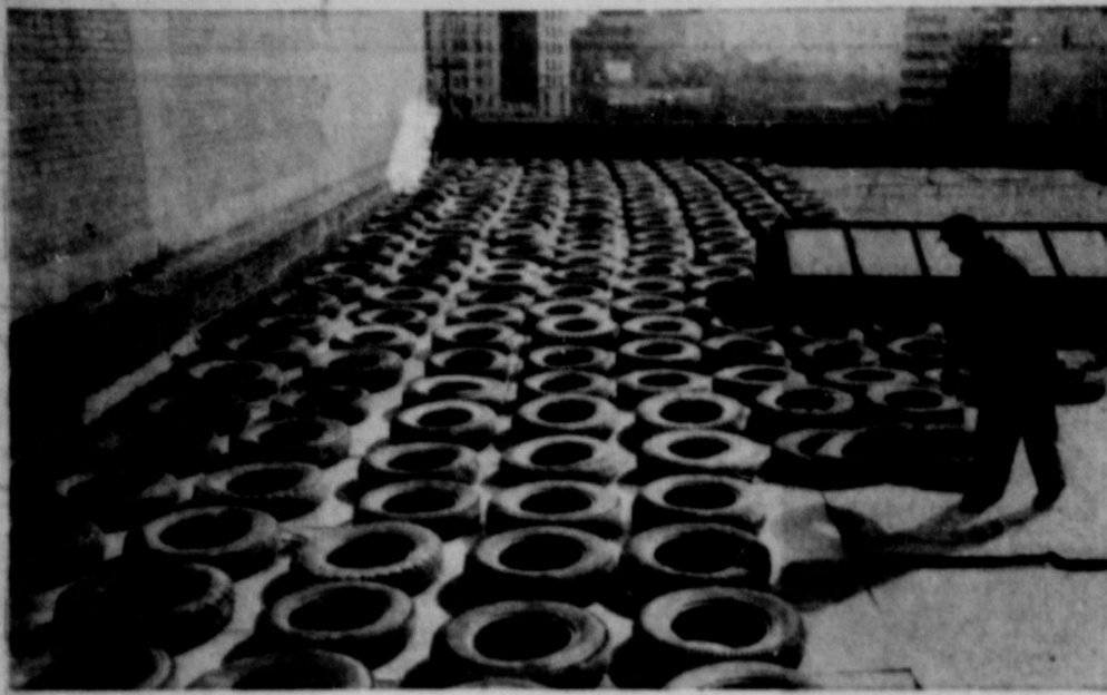
TIRING WORK—Worker lays down hundreds of rubber tires on a Rochester, N.Y., rooftop. The old tires are plywood sheeted and are used as protection against falling debris from the adjacent building being torn down.
