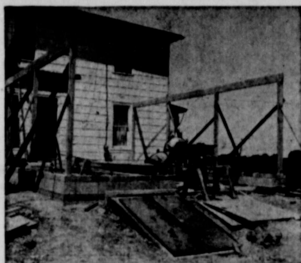
DUAL PURPOSE fallout shelter and carport-patio is shown under construction at the farm of John Holden near Hickory Corners, Mich. The shelter, to be used also for food storage, cost $1,200. With the carport and patio now being added, the cost totaled $2,300. Holden's family of three, and eight neighbors, gave the shelter a realistic workout recently when a small tornado struck nearby. An entrance to the shelter is in the foreground. (OCDM Photo)
