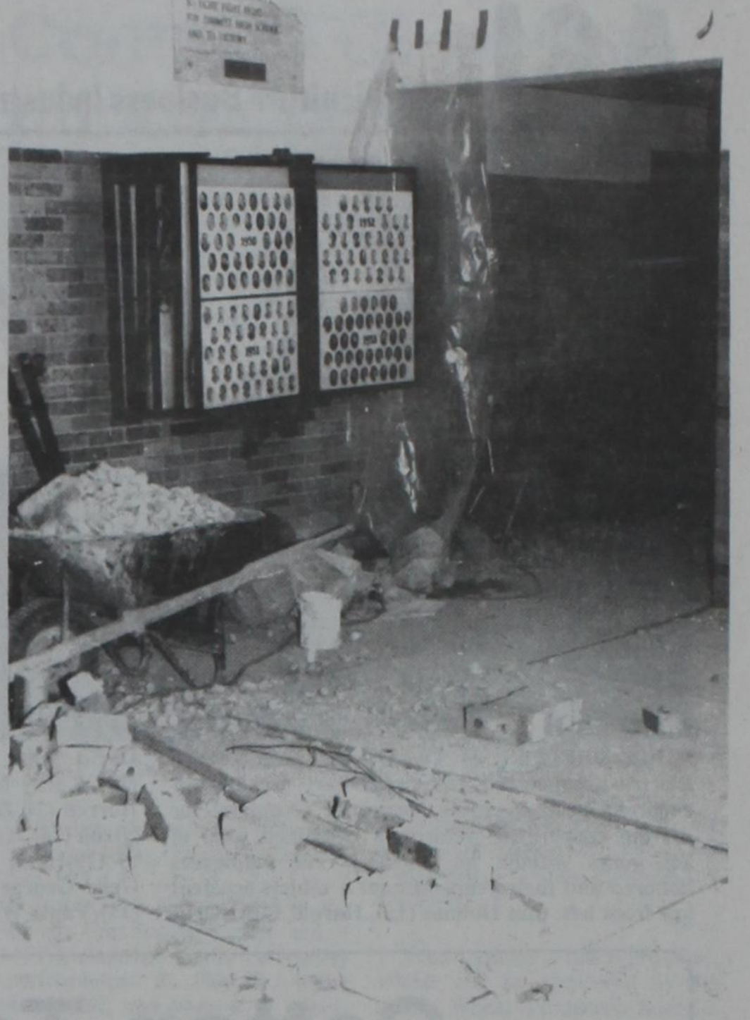
ALMOST FINISHED —Although some bricks and mortar remain in the high school's foyer, Assistant Principal Lyman Schroeder said the remaining construction won't affect classes, which begin Aug. 26. All exterior work is completed, and the construction crews are now detailing the interior, he said. Schroeder said every teacher should have a classroom by the first class day.
