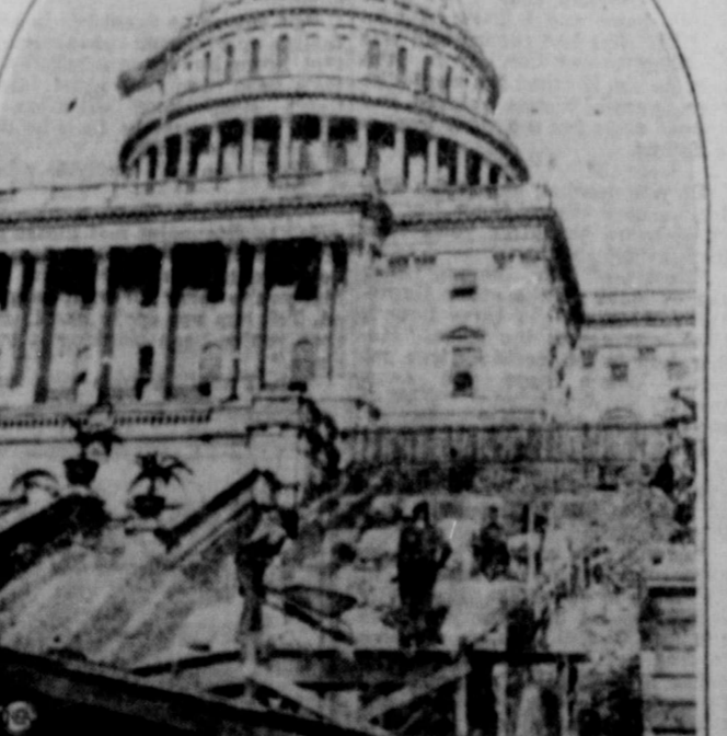
Worn out by the tread of sightseers, politicians and other visitors during the past 60 years, the stone steps on the west front of the national capitol at Washington, D. C., are being replaced, and here you see a crew of men at work. Brick work supporting steps against the capitol terraces is also being rebuilt.
