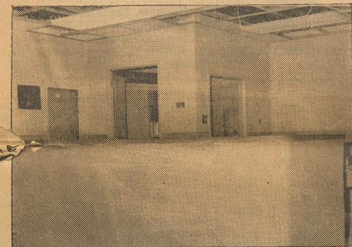
THIS PICTURE offers an inside view of the new hospital nursing station. Construction company announces the completion date of Plains Memorial will be about April 15. See story for details. —Staff Photo
