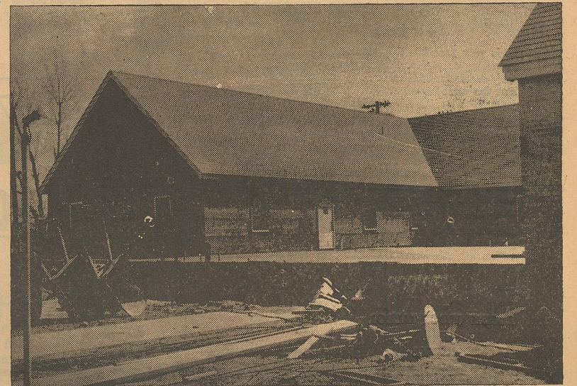
THIS VIEW of the Bedford Street Church of Christ shows part of the construction now underway which will result in an extension of the present education and worship facilities. See story for details. —Staff Photo
