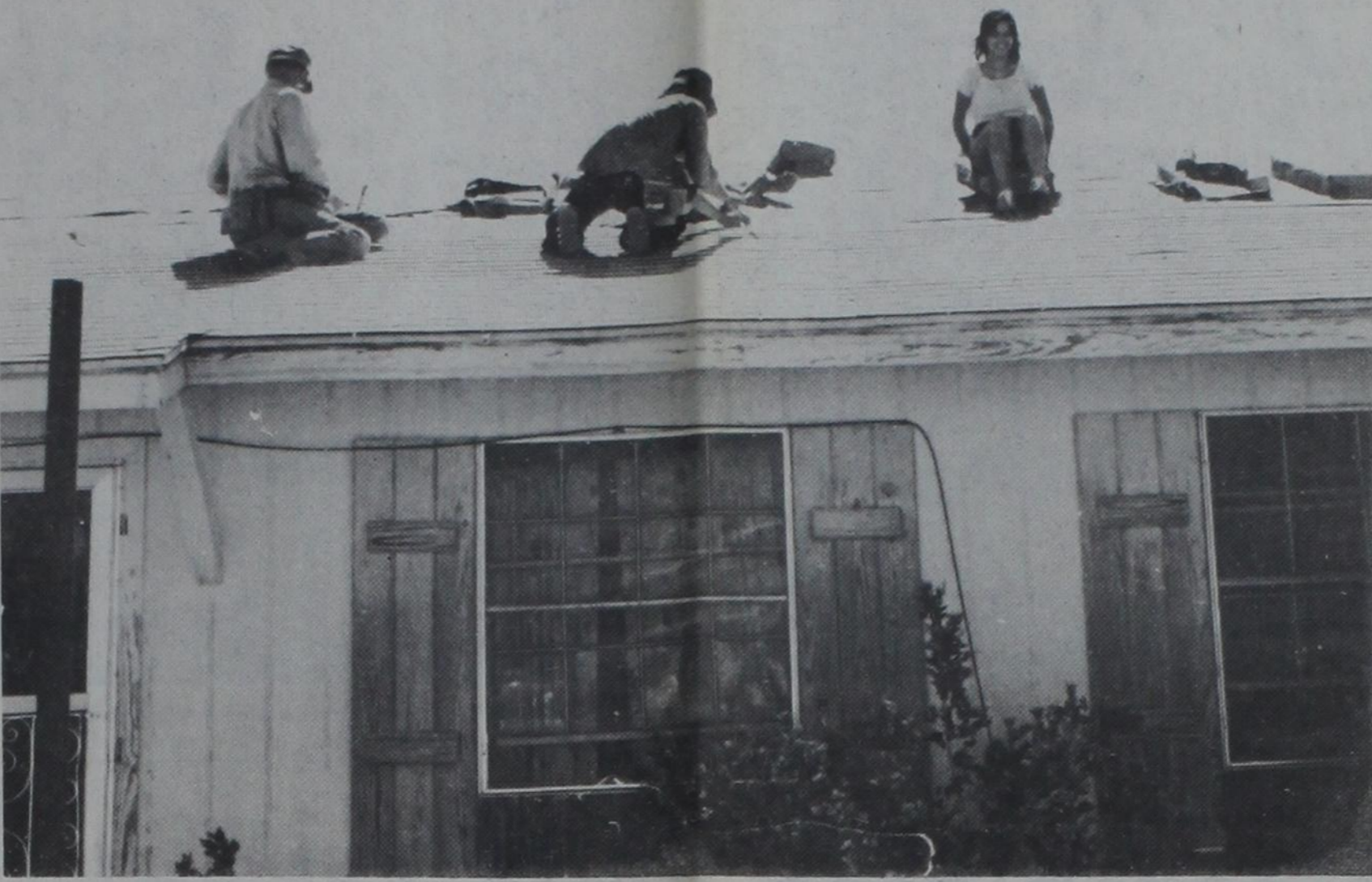
FAMILIAR SCENE—There's a lot of activity at rooftop level in Dimmitt this week as appraisers and roofers work to repair the damage caused by the May 28 hailstorm. This scene at the
