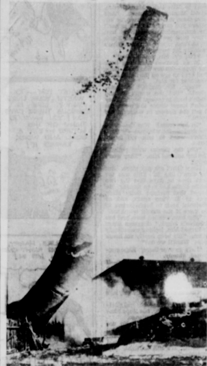
Down to earth crashes this 35-year-old, 135-foot stack at Norway, Michigan, caught by camera just after powder blast ripped out its foundation.
