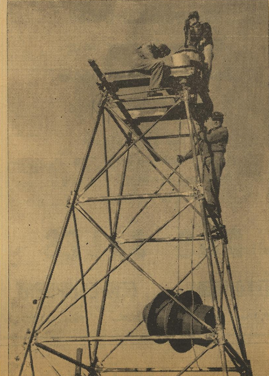
CITY EMPLOYEES (left to right) Buck Raper, Howard Grand and Richard Woods install the new fire siren. They are hauling the bright red cover for the siren in completing the installation Thursday morning. See story. —Staff Photo
