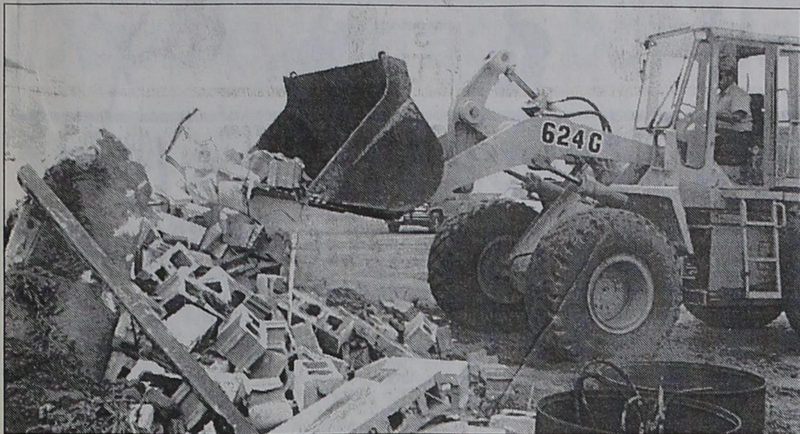
KNOCKING IT DOWN —The old 700-sq. ft. center block office at North Gin of Dimmitt, which was constructed in 1956, was burned and then knocked to the ground April 12 to make way for a new, larger building on the same site. According to gin manager Jim Bradford, construction is expected to start this week,
