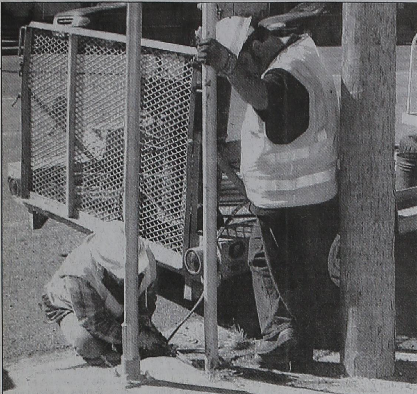
GETTING SOME WORK DONE — These Highway workers are shown doing some highway sign work on Bedford Street.
