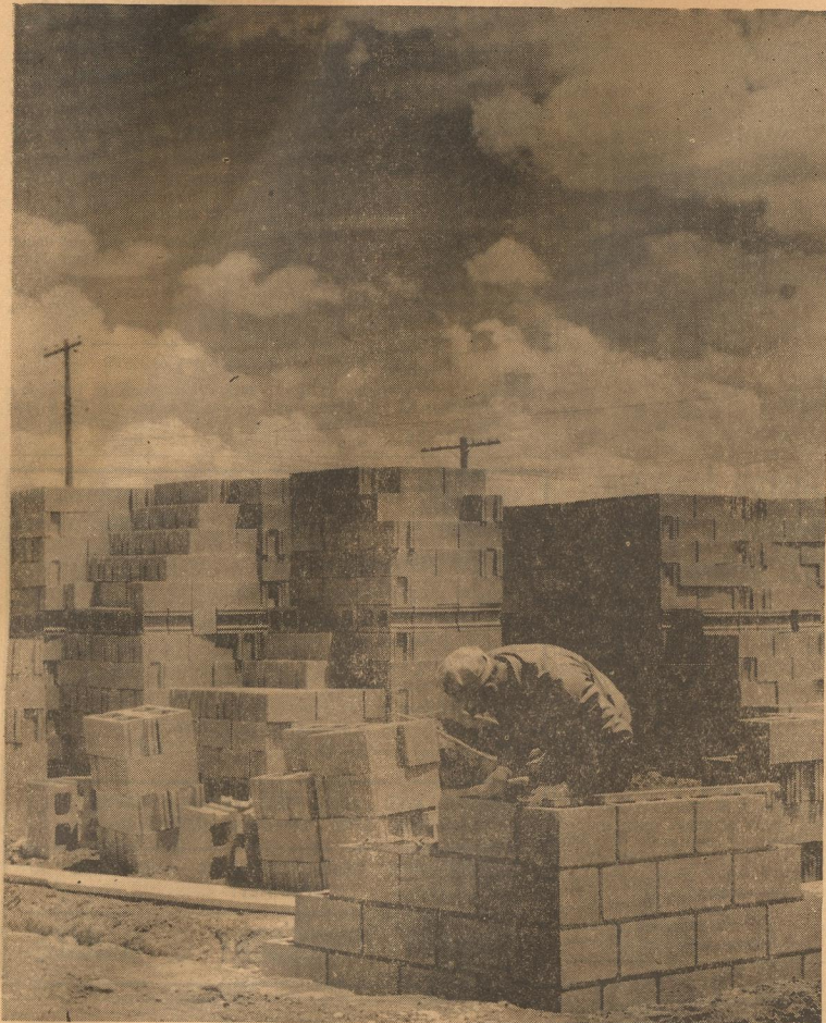
NEW SHOPPING CENTER under construction across the street and north of the post office is being erected by Paul Acker Builders under the direction of its owner, Ray Bearden. Shown laying concrete blocks for the walls is Clarence Moyer, a Paul Acker employee. —Cowan photo
