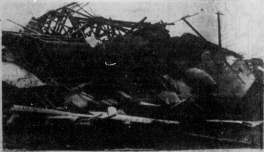
All that remains of a huge cotton gin at Port Lavaca, Texas after the hurricane passed was this pile of debris. Many homes were destroyed and property damage was high. (NEA Telephoto.)
