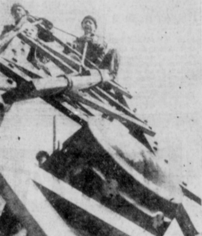
Cameraman perched 102 stories above Manhattan's streets got this picture of workmen installing new television antennae atop the Empire State Building New York City. The photographer said the height didn't bother him, much. (NEA Telephoto.)
