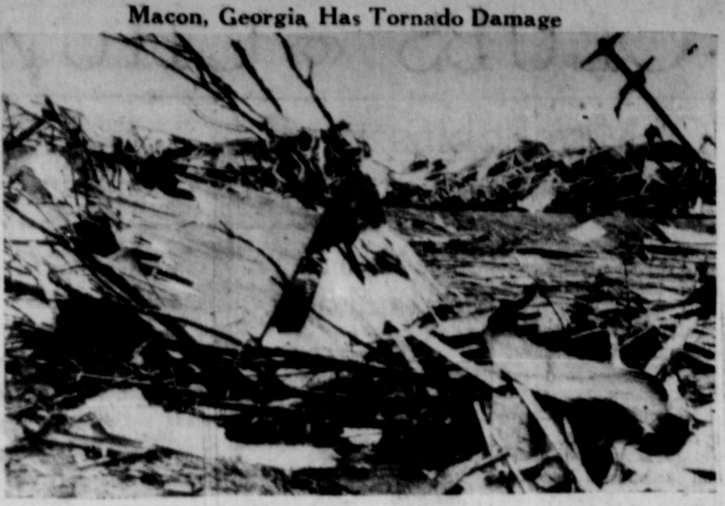
Macon, Georgia Has Tornado Damage A tornado, ripping through the Macon area, tore down an Army hanger at the Air Base adjoining Camp Wheeler. No one was in the building at the time, but you can see by the wreckage that the damage was quite complete. (NEA Telephoto).
