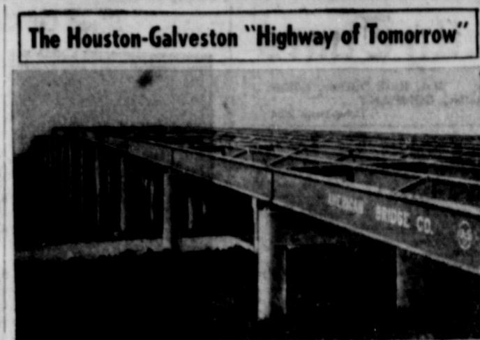
The Houston-Galveston "Highway of Tomorrow" This rising steel and concrete structure over Calhoun Road in Houston, Texas, will carry the heavy traffic of the new Galveston-Houston express highway through the Texas metropolis' booming East End. A 1,192-foot structure, this overpass comprises one of five in Houston's East End, the steel for which is being furnished by the American Bridge Company, subsidiary of United States Steel. The 50-mile expressway, termed among highway builders as "the highway of tomorrow," will be the ultimate in new highway construction in Texas, a state already famed for its fine highway system.
